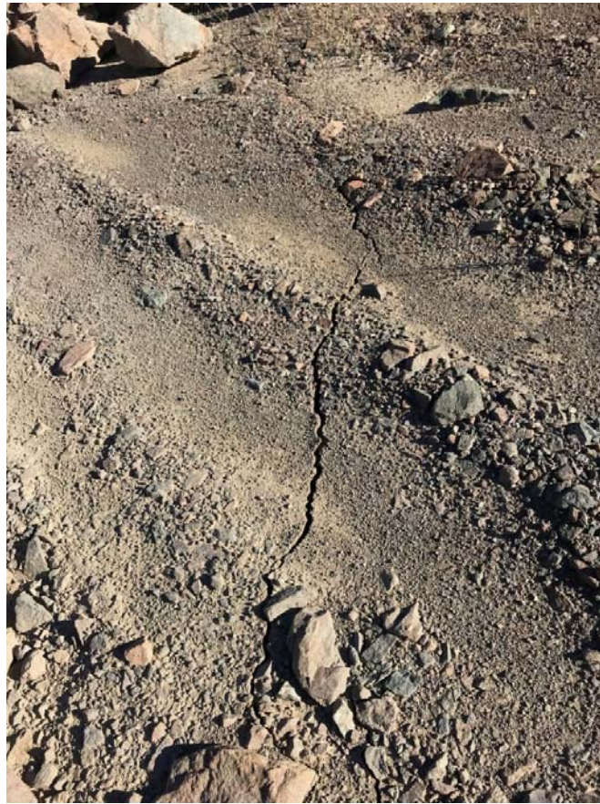
Figure 3-14: Photograph of cracking on the Stage 5 crest beside Standpipe P9 taken at 07:48, March 9, 2018
