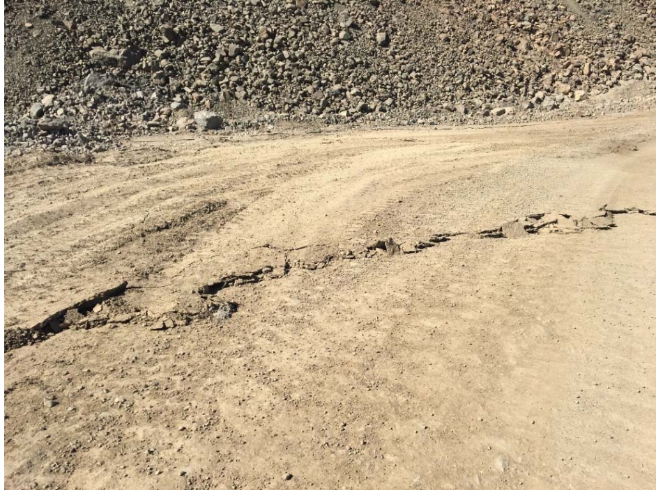
Figure 3-16: Cracking and heaving of haul road at Chainage 2060, March 9, 2018
