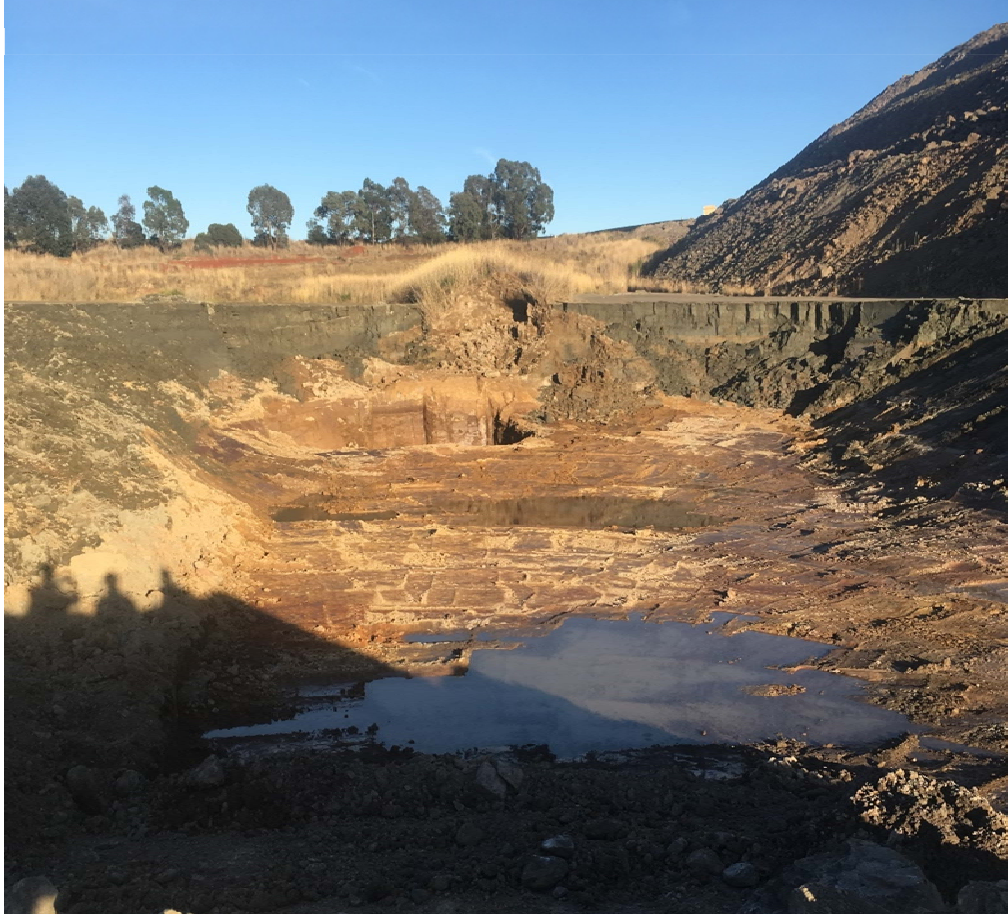
Figure 3-7: Exposed foundation on January 18, 2018
