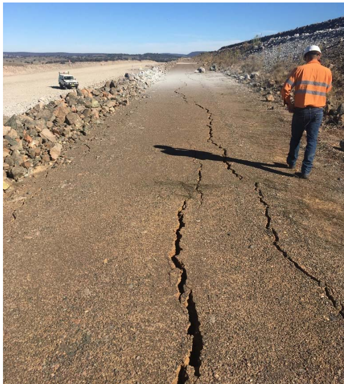
Figure 3-15: Stage 8 crest cracking looking west, March 9, 2018
