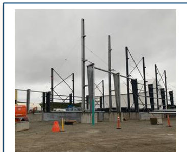
Continue to upgrade facilities, with the construction of life of mine maintenance and combined office buildings
