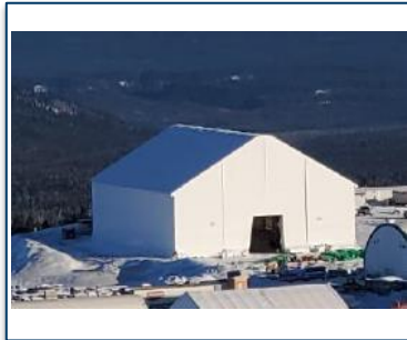
Improved working conditions for Red Chris employees with temporary workshop & long term warehouse
