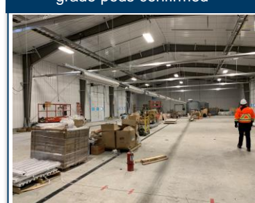
Permanent long term core processing facility nearing completion for CY21 field season
